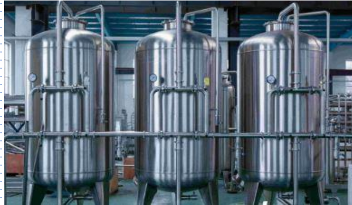
Filter system for mechanical water purification
